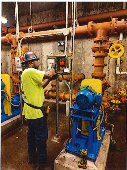
Figure 4: New RAS Pump
